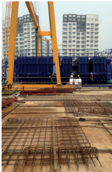
In the foreground: prepared reinforcement cages In the background: the compact mobile battery mould (MBM)
